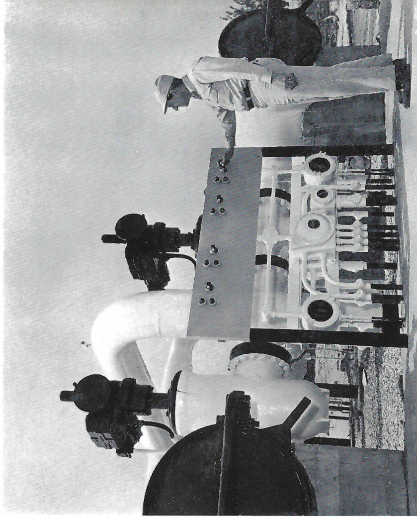
All shipments pass through strainers and excelsior-filled "hay tanks" as they enter the line at Kennedy station. Here the operator pushes a button to switch "hay tanks" for cleaning. The equipment below the panel consists of electrical safety devices which automatically take a unit out of service if an abnormal operating condition occurs.
