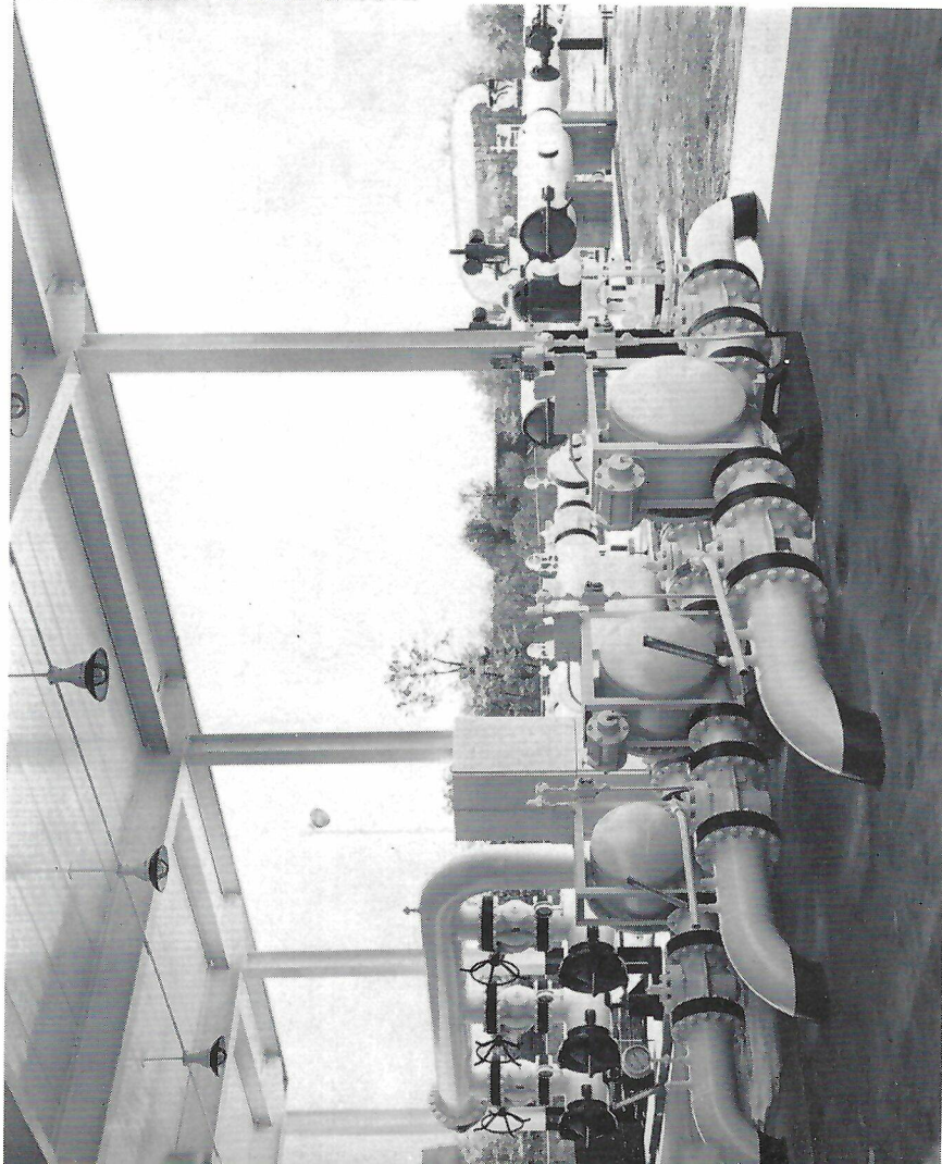
All shipments are measured automatically by meters as they enter and leave the Wolverine line. Above is the metering manifold at Kennedy station, with strainers in the background.
